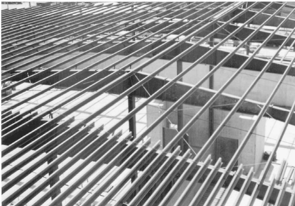
FIGURE 5.10 Two additional simple-span purlins are placed between continuous purlins in the end bays of this building.
